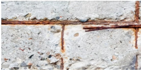
Figure 2.27: An example of calcium chloride effect on the reinforcement, adapted from https://fritzpak.com/
