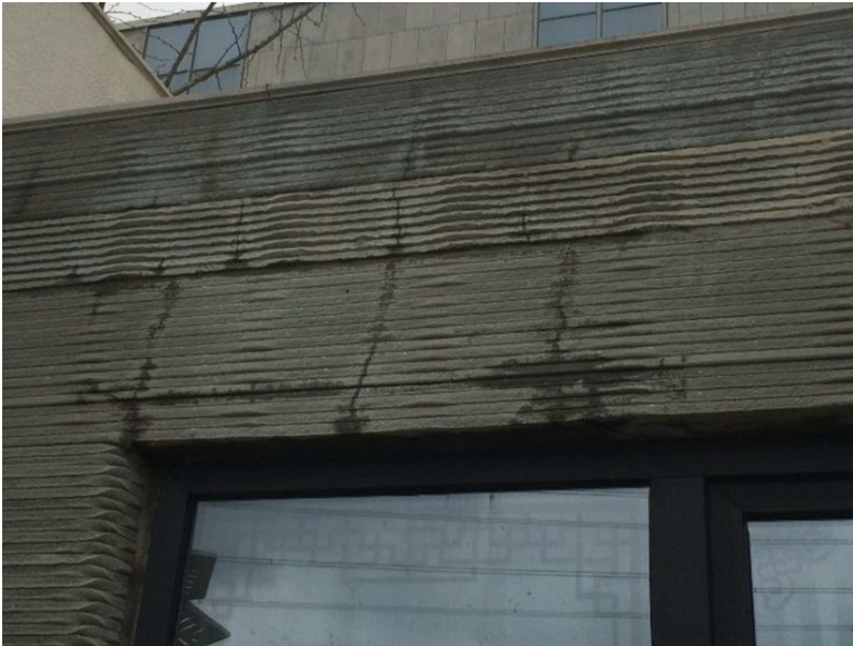
Figure 2.12: Interfaces between printed concrete layers and cracks show evidence of local capillary suction, photo by V. Mechtcherine, adapted from [52]
