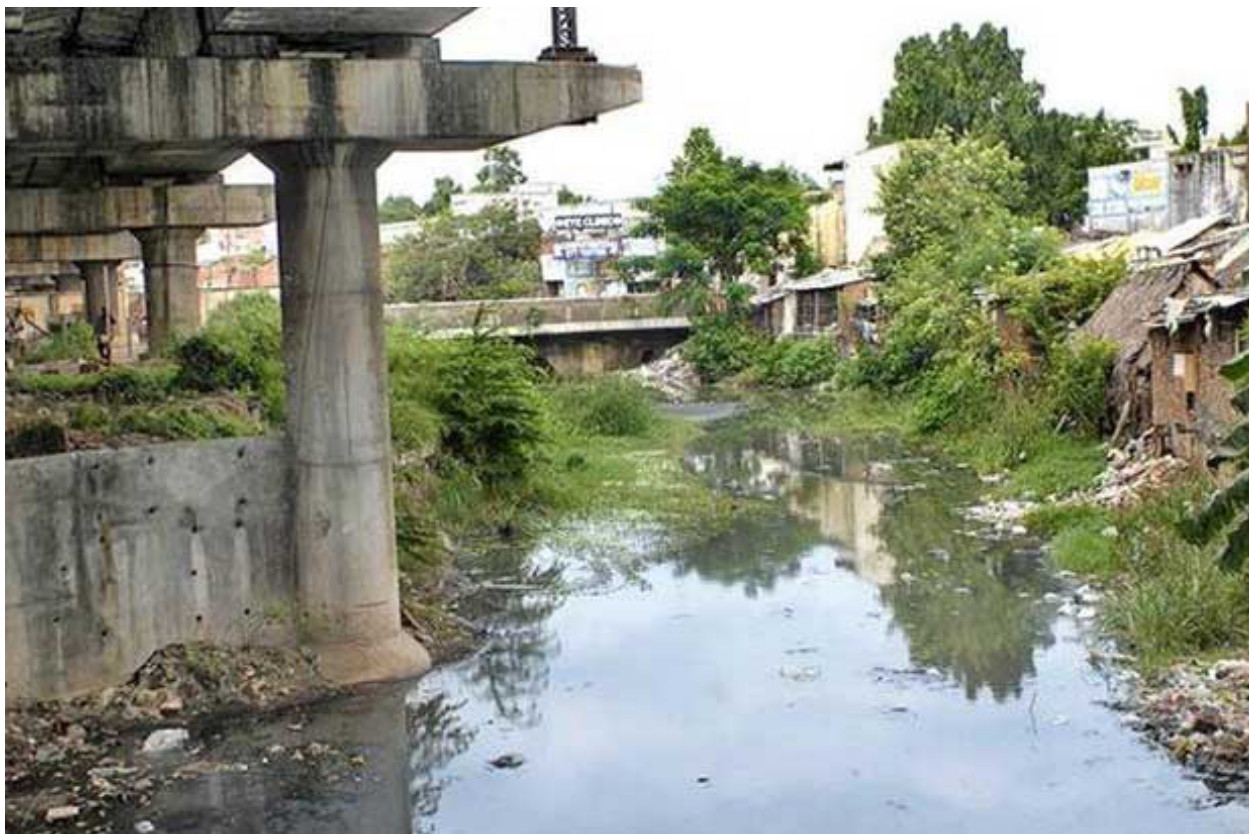
Mobility infrastructure encroaching Buckingham canal
