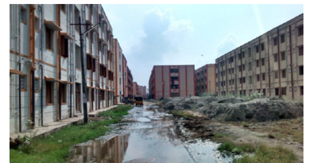
Figure 4: TNSCB resettlement tenements at Ezhil Nagar seen flooded with sewerage water: a sorry state of affairs. Retrieved from https://www.cag.org.in/blogs/when-poor-have-no-voice-brief-summary-hearing-national-green-tribunal-case-related-cooum .
