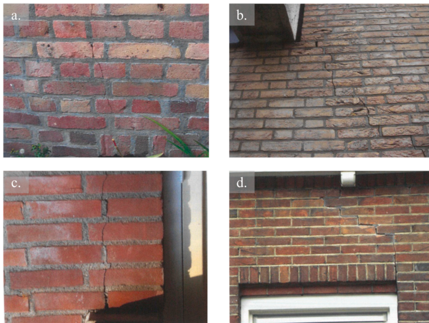
Fig. 3. Photographs of cracks in bare masonry walls. (a) Small crack narrower than 0.5 mm; (b) crack approximately 2 mm wide; (c) crack narrower than 2 mm; and (d) wider than 5 mm. Adapted from SBR [60].
