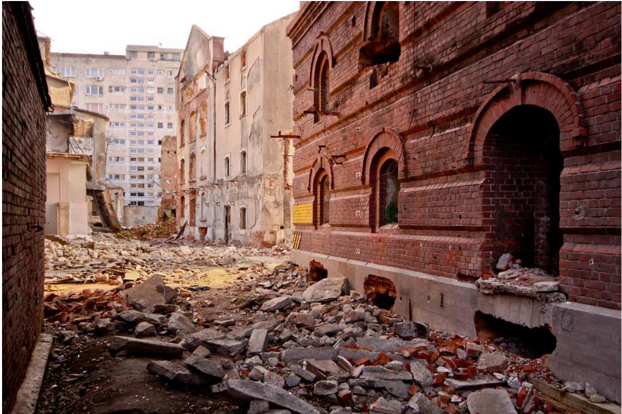
Figure 24. Photograph of Assan's Mill degradation, 2019
