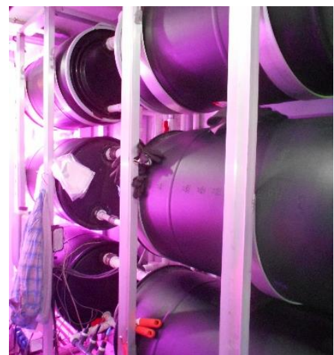
Figure 12 Built-in water storage
