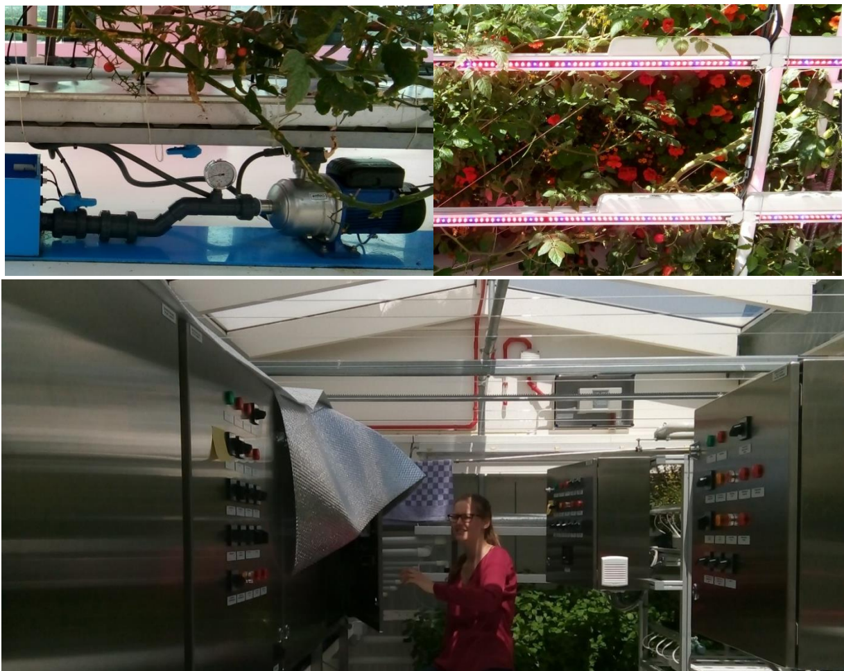
Figure 8 Electricity consuming technologies in the greenhouse: pumps (top left), LED lights (top right) computer operation system(bottom)
