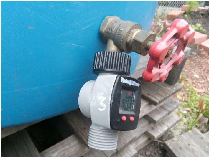
Figure 21 Water meter attached to the garden hose outlet of one of the rainwater barrels
