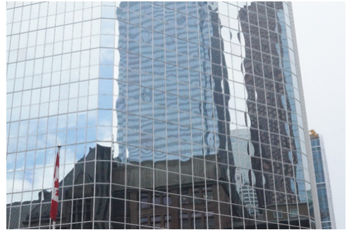
Figure 3.2.1.2: Appearance of deformation of glass panes Source:own illustration.
