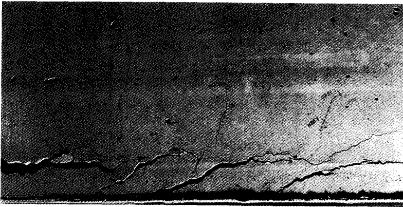
Fig. 5.20 Concrete cover between internal bars and steel plate; concrete struts are visible
