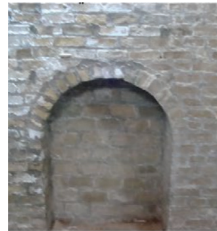
Opening in the Nim double wall. image by Kammunah, The impact of architectural heritage on the development of Najafi architecture.
