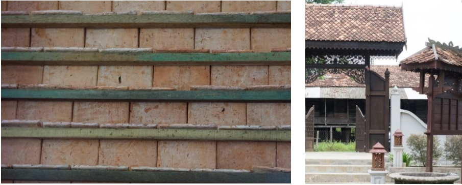
Figure 10.8: Stacks of Atap Singgora (left), view of the tiles from inside (middle), the tiles in combination with structures with traditional wood carvings (right).
