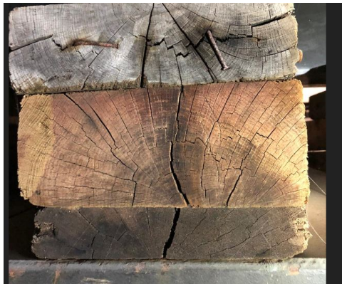
Figure 6.2: Cracking failure mechanism
