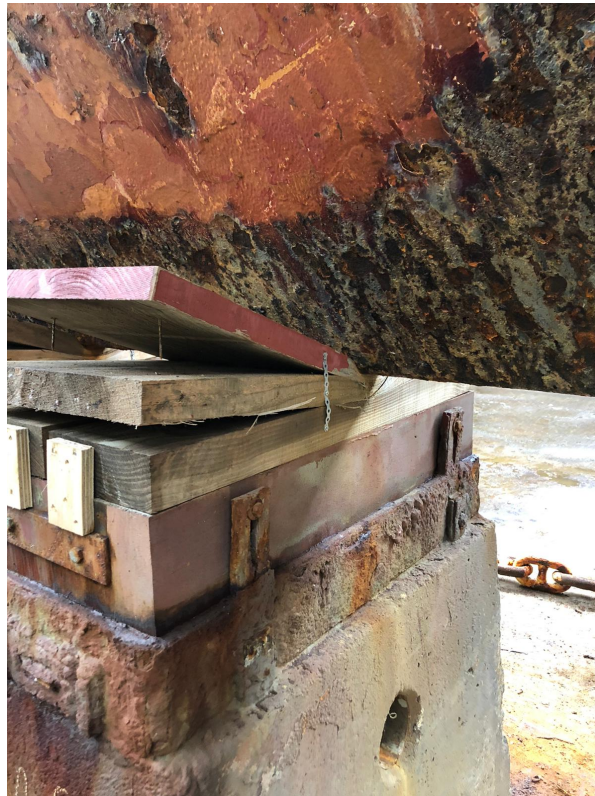
Figure 1.1: Over-stress failure due to a minimized contact area in the fore of the ship. Complete failure of the softwood is the consequence of the small contact area. (DAMEN yard, Ritthem)
