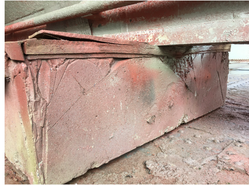
Figure 2.15: Stellendam dock block (damage)
