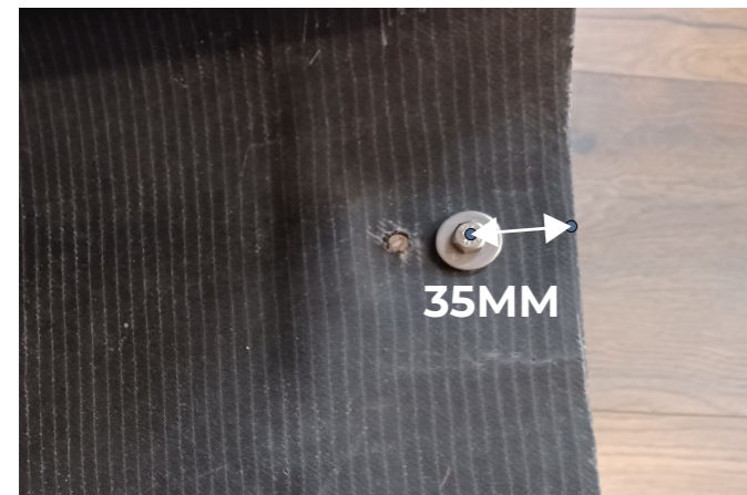
Figure A-5.6: distance between bolts and end of seat (35mm, measured from center of hole)
