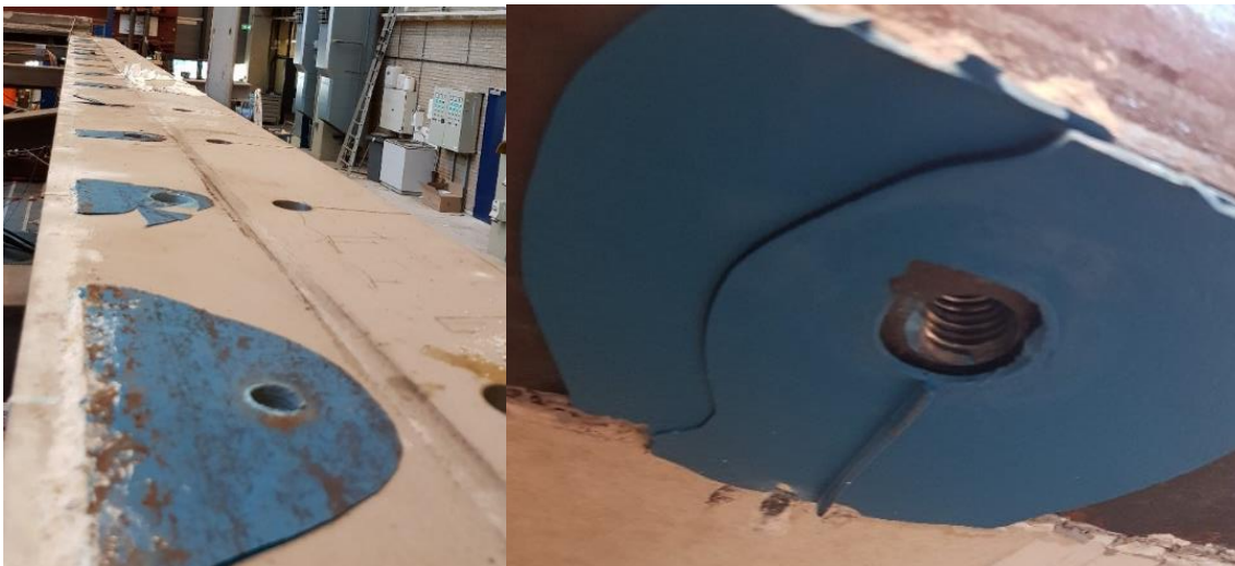
Figure 3.59 Leaked resin on top flange and deck
