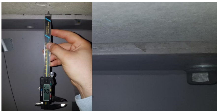
Figure 3.57 Gap between deck and top flange before and after tightening the bolt
