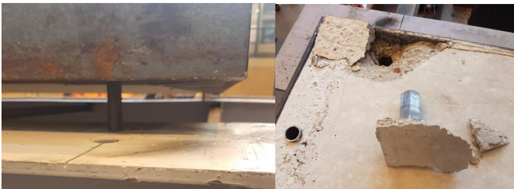
Figure 3.15 Damage due to supported deck on threaded rods
