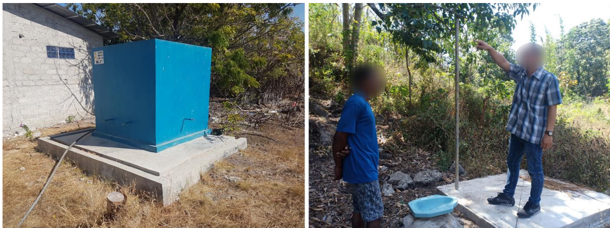
Figure 1. Examples of unsustainable WASH services in East Sumba. Left: A not functioning water tank; Right: An unfinished latrine construction. Pictures were taken by the first author.
