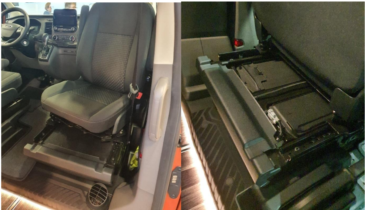
Figure K.19 Placement of the batteries
