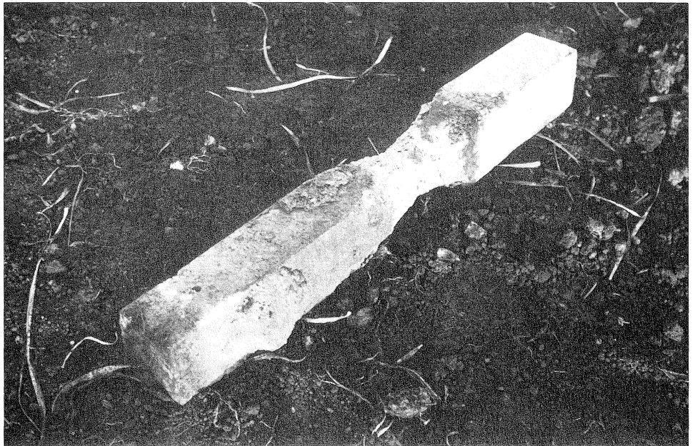
Fig. 9. Deteriorated greenhouse foundation pile (12).
