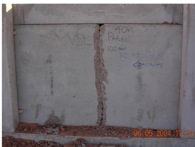
Figure 7.6: Panel 4 after the blast
