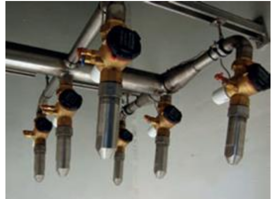
Figure 11: The 9 water spray heads of the Climate Cascade at The Four Elements hotel. Source: Heirbaut, 2019.
