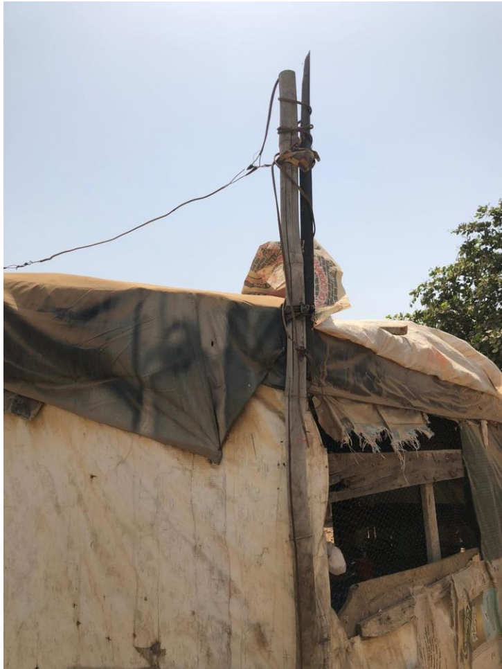
BAMBOO POLE FOR CONNECTION TO ELECTRICITY
