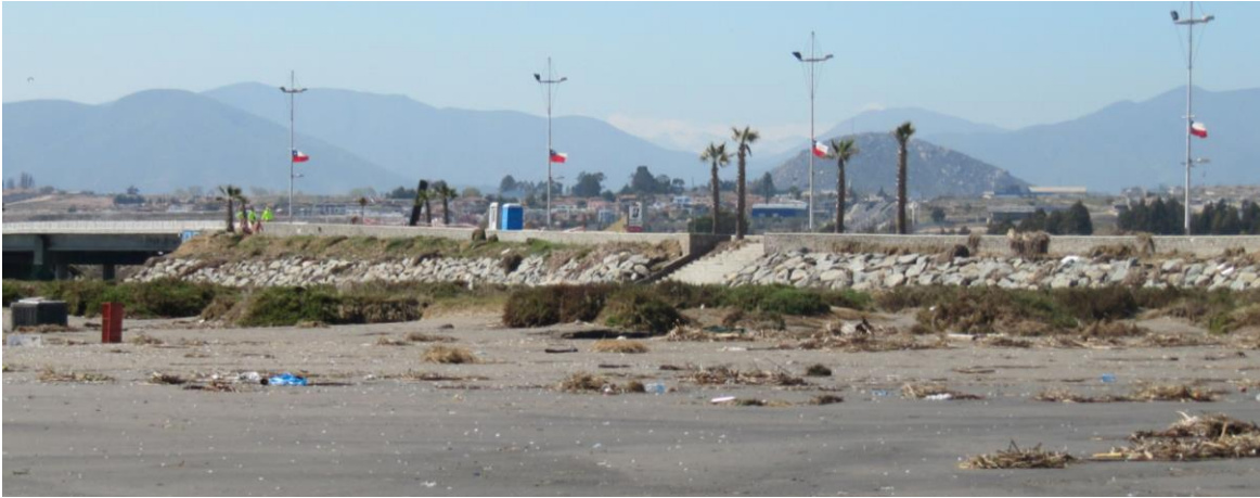
Figure III - 10: Road with bridge, minor damage (still usable road and revetment).
