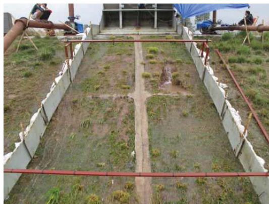
Fig. 7. Damages initiated at existing holes, Thai Thuy dike, Thai Binh province.
