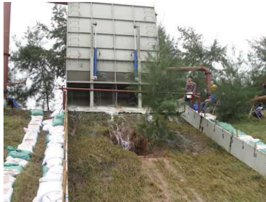
Fig. 6. Damage at a tree on the grass slope, Thinh Long dike, Nam Dinh province.
