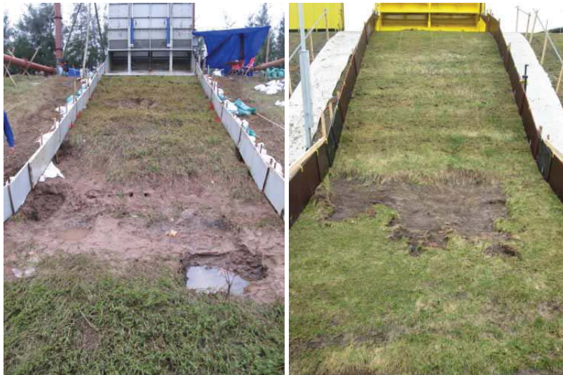
Fig. 5. Damages at transition between the steep part and the horizontal toe, left: Think Long dike and right: Afsluitdijk.
