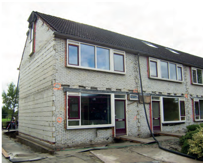
Figure 5.3: Stripped terraced house with the outer leaf removed before placing the steel frame in the cavity. [10]
