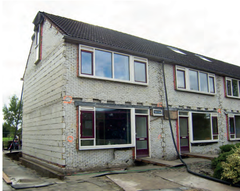
Figure 1.5: Stripped terraced house with the outer leaf removed before placing the steel frame in the cavity. [10]
