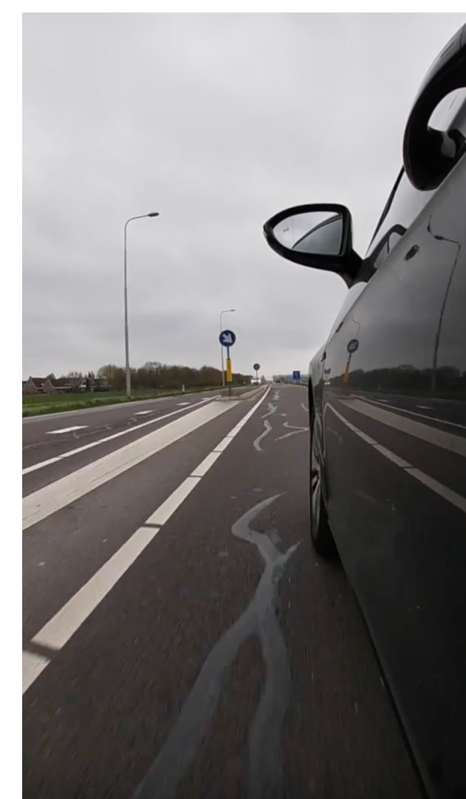
Asphalt repair patches
