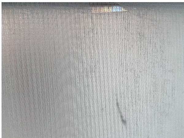
Fig 8.7: Spot missing peel ply and smudges
