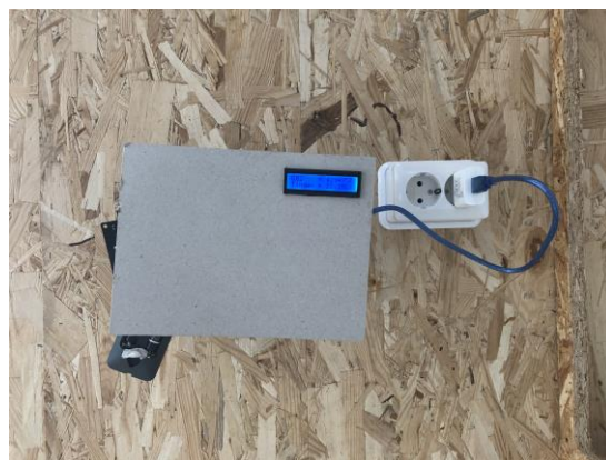
Figure 4-21 Controller mounted on the ceiling of the PDLab
