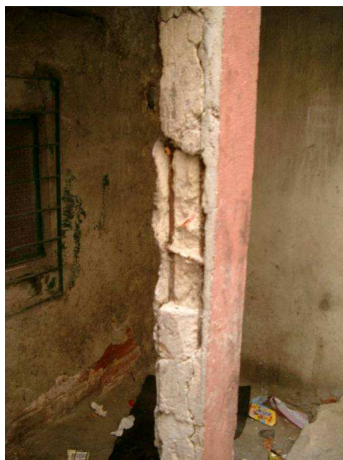
Figure 4. Column with detached concrete covering and insufficient transverse reinforcement.
