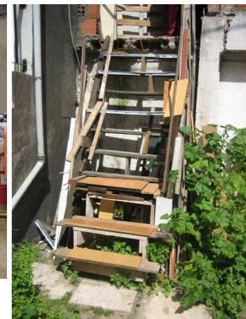
Figure 6. Stairs of poor construction quality.
