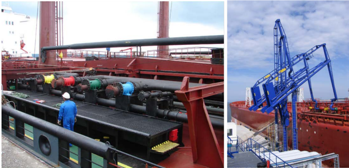
Figure 5.3: Liquid bulk (un)loading facilities; left: manifold ( Maya OBO carrier 3 by Herv Cozanet is licenced under CC BY-SA 3.0); right: (un)loading arms ( Marine Loading Arm KLEa by Ljl.kanon is licenced under CC BY-SA 3.0).
