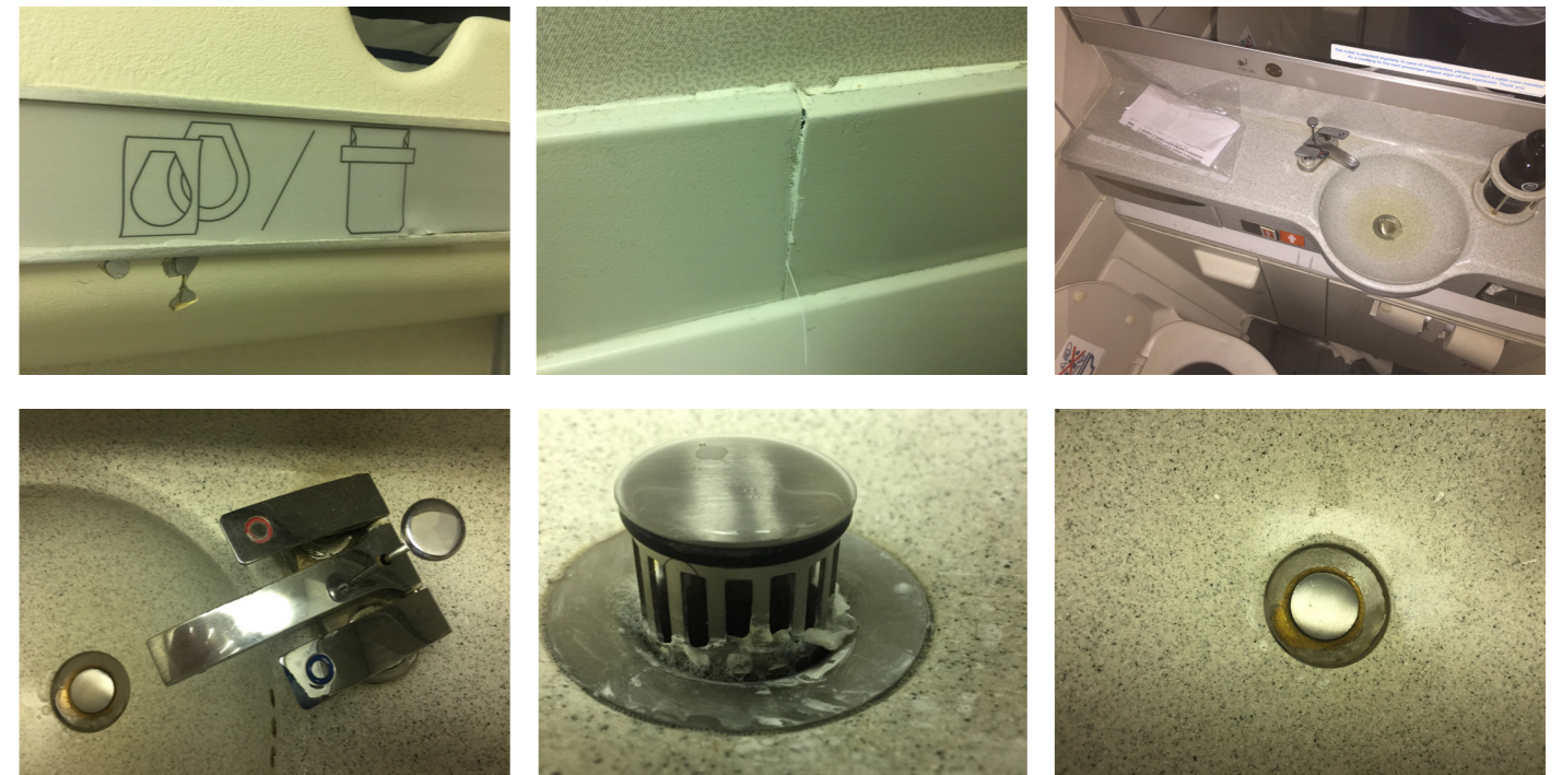
Fig.4.01-06 Damage, discoloration and water scum
