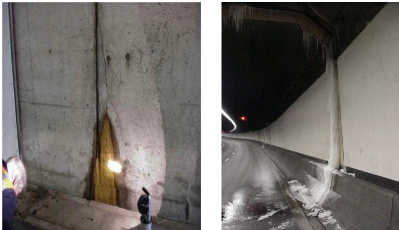
Figure 1.8 - Water leakage in the connections of the Kiltunnel (left) and Drechtunnel (right) [3]
