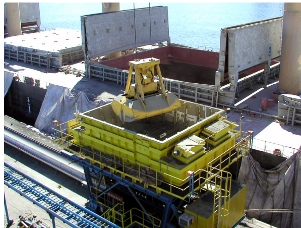
Figure 3.5: Ship unloading into a hopper before it is loaded on the belt conveyor [25]
