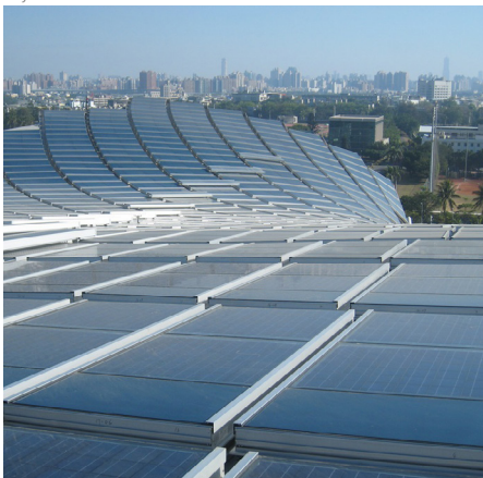
The roof of the Dragon Stadium designed by Toyo Ito powers the whole stadium. It also gives shading to the visitors on sunny days.
