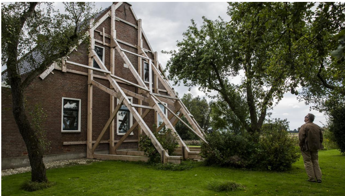
Figure 2.7 Earthquake damaged dwelling at Groningen (KNAG, 2016)
