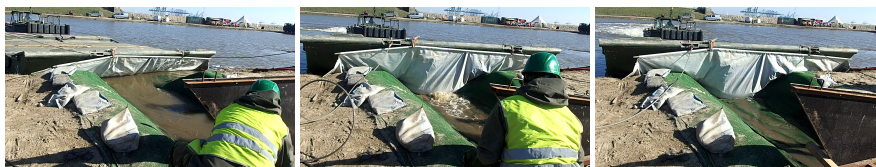
Figure 3.22: Dynamic placement of the BresDefender at Hedwigepolder. From left to right: pontoon at the breach before opening the hatch, pontoon during impact levee and pontoon after adjustment of the tarpaulin
