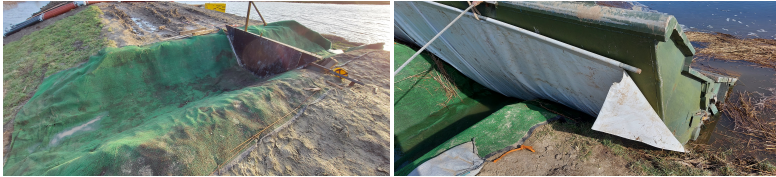
Figure 3.7: (left) Weir to regulate water through breach, (right) BresDefender with white tarpaulin
