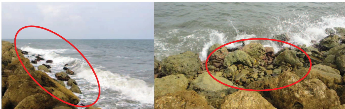
Figure 3.13 Loose rocks have come off the seawall slope (left) and exposure of underlying smaller rocks (right)
