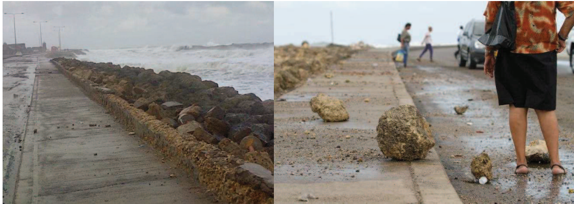
Figure 3.14 Storm conditions (left) damage to sea wall due to storm (right)
