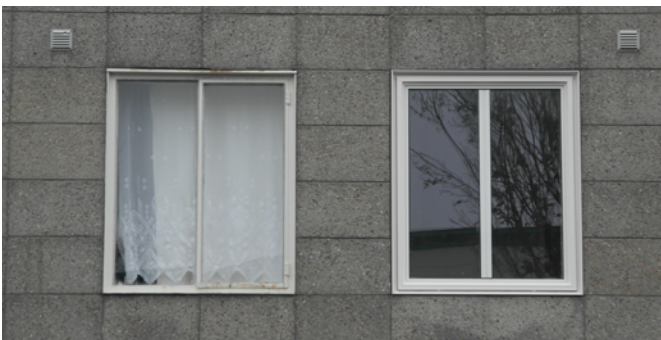
Amount : strip (A) 111 / strip (B) 132 Material : Steel (original) / Aluminum (new) Size : 1250 x 1500mm
