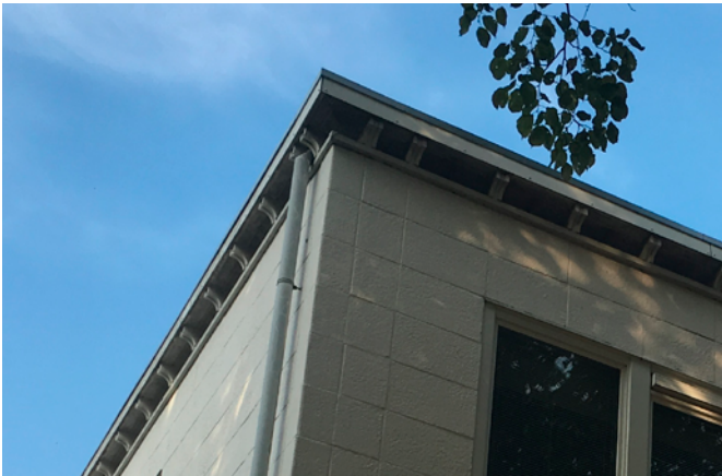
Amount : strip (A) 192 / strip (B) 222 Material : Wood (roof gutter) Size : N/A
