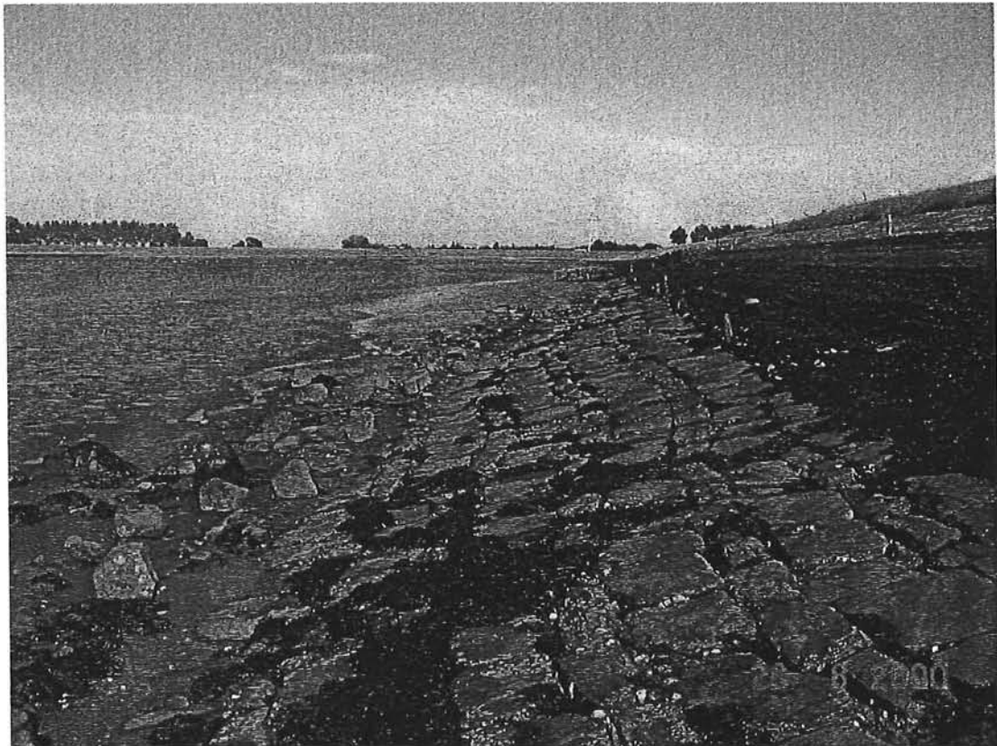
"Doornikse" blocks (an old type of pitching)
