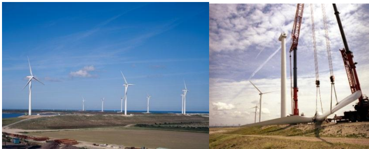
Figure 61 ... (left) Overview of the Windpark Slufter (right) A wind turbine assembling at Windpark Slufter ( Eneco, 2006 )
