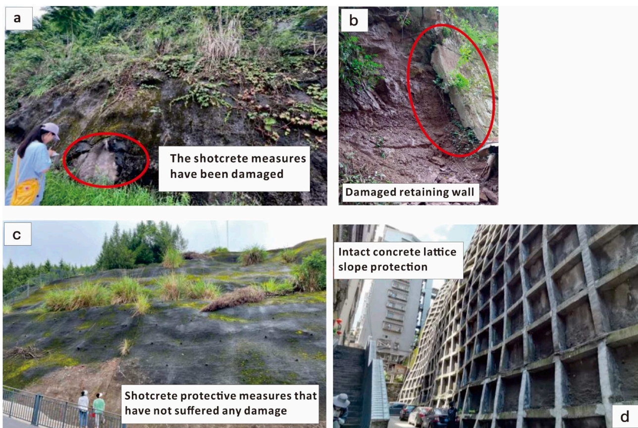
Figure 13. Field survey of protective measures ((a,b) damaged “partial protection” measures; (c,d) intact “more protection” measures).
