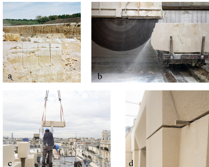
Figure 5. Key steps in construction of the Social Housing Project by Barrault Pressacco.
