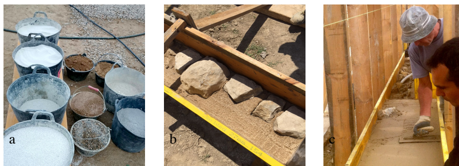
Figure 10. - Photos showing the process of making the Casa 1413 stone rubble cast walls
