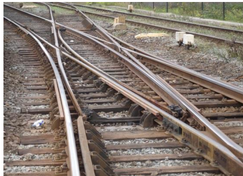
Figure 9.20 Example of a double switch
