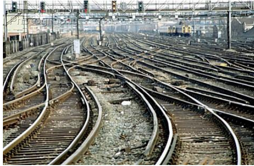
Figure 2.2 'Tangled' tracks at London Bridge station
