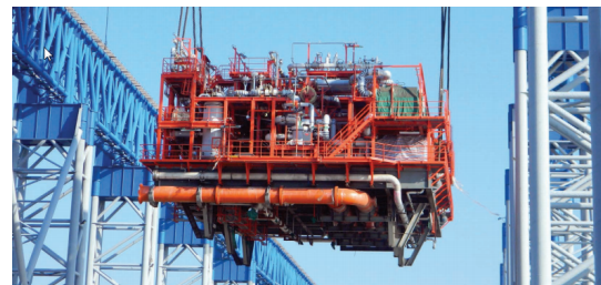
(b) Installation of the system onboard of the vessel "Nusantara Regas Satu" [15]
