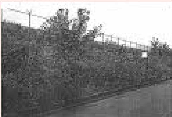
Figure 98: The steeply sloping embankment of the Metra rapid transit rail line. This is the situation with overgrowth of ruderal vegetation (Gobster, 2010).
