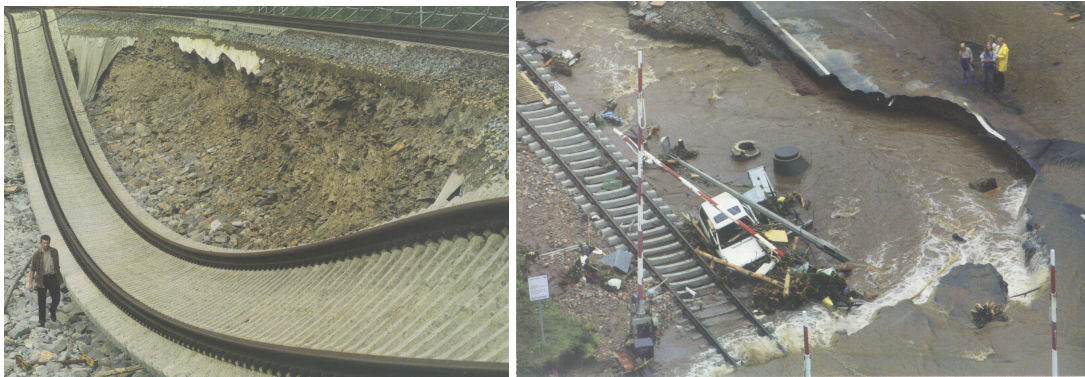
Figure 5 Scour of railways and roads
