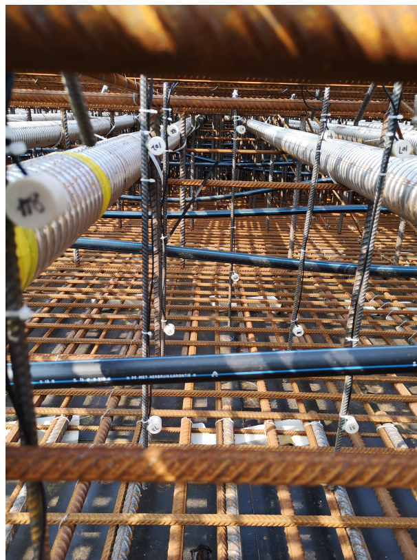
Figure 1.2: Positioning of smart aggregates in the formwork of a cast in-situ bridge under construction (Yang 2021).
