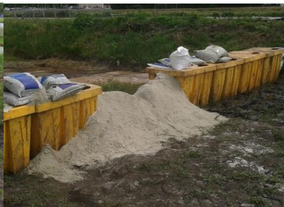
Figure 6.3: Depression in the sand dike
