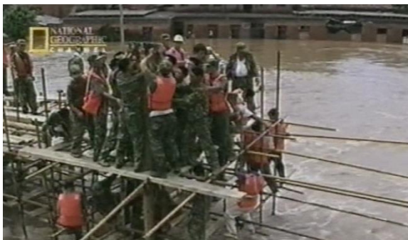
Figure 4.22: Construction of scaffolding to close the breach (Rage of the River Gods, 2001)
