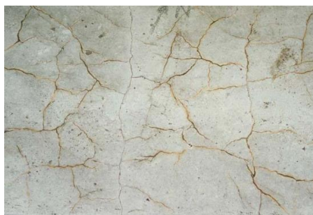
inhomogeneous anisotropic cracks Map crack pattern
