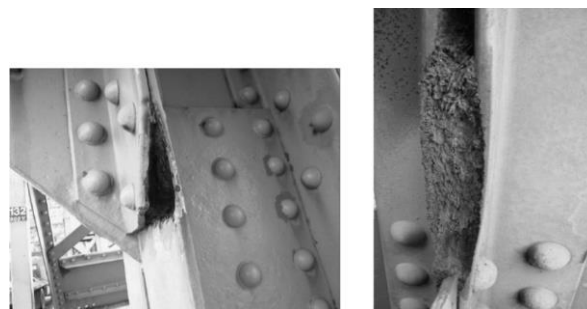
Figure 68: Delamination due to corrosion around the scribe
