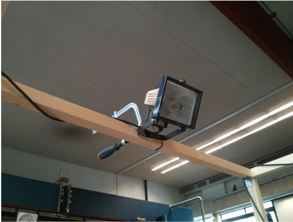
Figure H.3 – Light attached to wooden frame above flume
