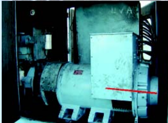
Figure 6: Generator before refurbishment.
