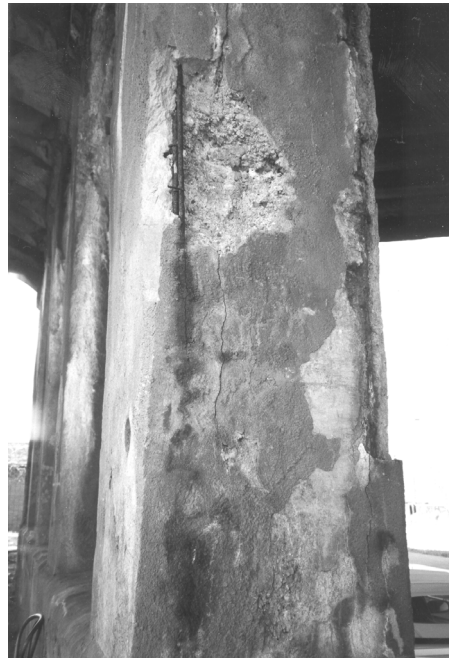
Figure 8: Corrosion process (Ann Arbor, MI, US, photo by author)
