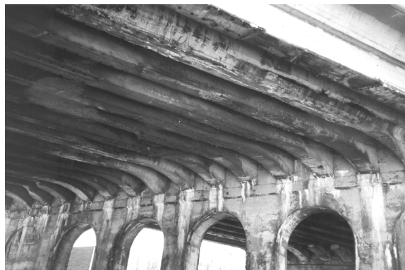
Figure 3: Deteriorated bridge, constructed in \pm 1915 (Ann Arbor, MI, U.S., photo by author)
