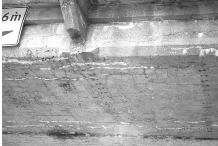
Figure 6: Damaging cracking and exudation of gel (Sherbrooke, QC, Ca, photo by author)
