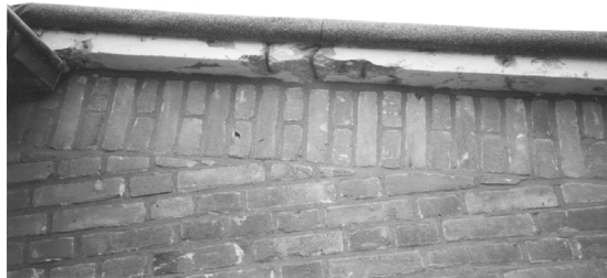
Figure 10: Corrosion due to carbonation (Bloemendaal, the Netherlands, photo by author)
