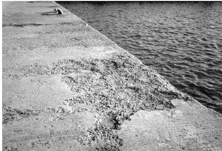
Figure 5: Freeze-thaw deterioration (Owen Sound, ON, Ca, photo by author)
