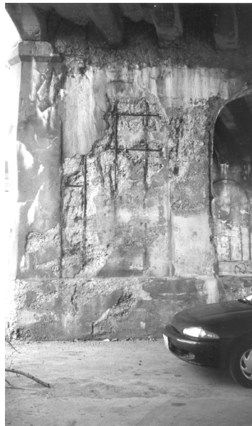
Figure 4: Severe spalling at bridge pier (Ann Arbor, MI, U.S., photo by author)
