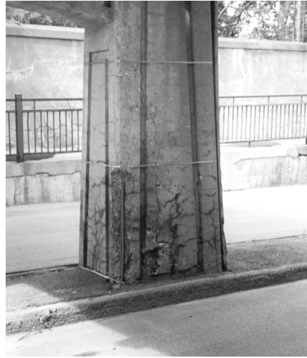
Figure 9: Corroded railway bridge column (Sherbrooke, QC, Ca, photo by author)
