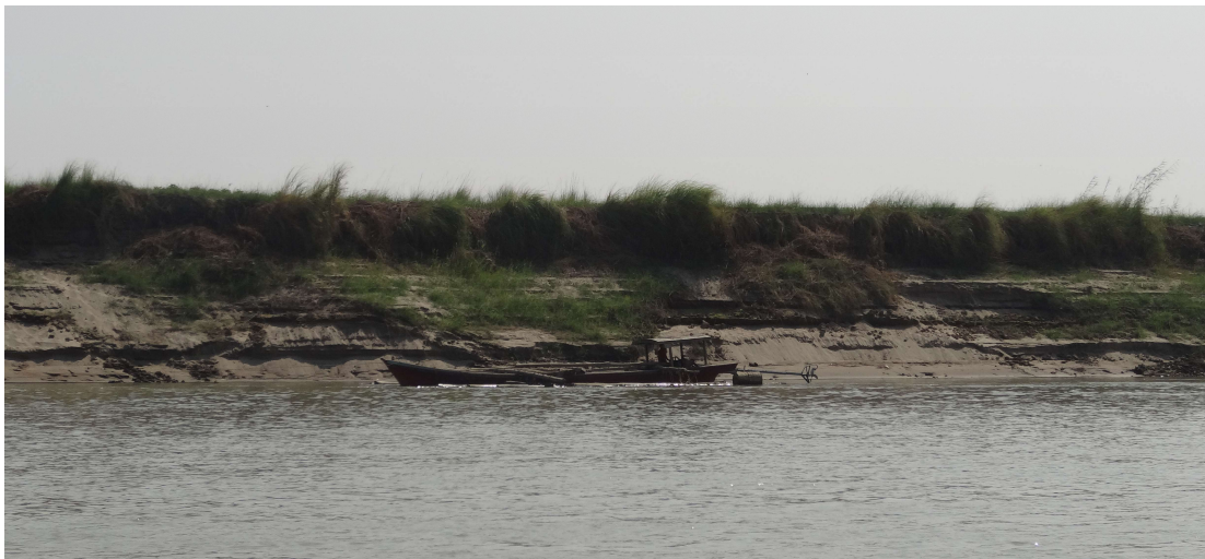
Figure 16 Shear plane failure is also evident in the Ayeyarwady river. The ridges on the bank indicate locations where shear failure has taken place.
