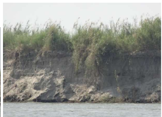
Figure B5 Grassy vegetation on this riverbank is not able to prevent toe erosion and mass failure.
