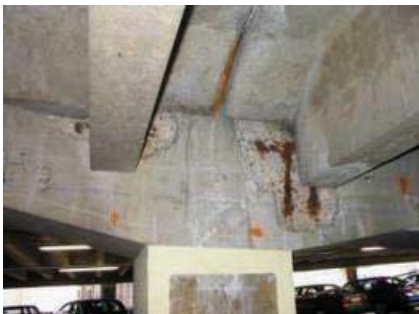
Figure 3.2: Uncovered rebar [CIE5127]
