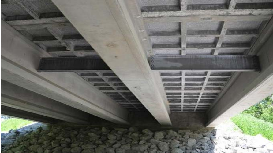
Figure 1.1: Little Cedar Creek bridge USA 2011, Ductal UHPC waffle deck, girders and joints
